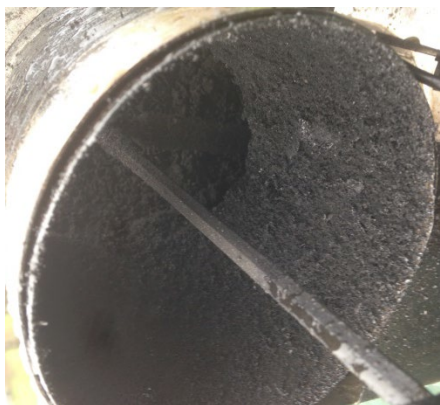
Black wood-coal soot, 4-10mm thick on upper flue wall, under 0.5mm on electrode, 27 June
