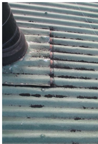
Particles on the roof from the wood-coal fire
