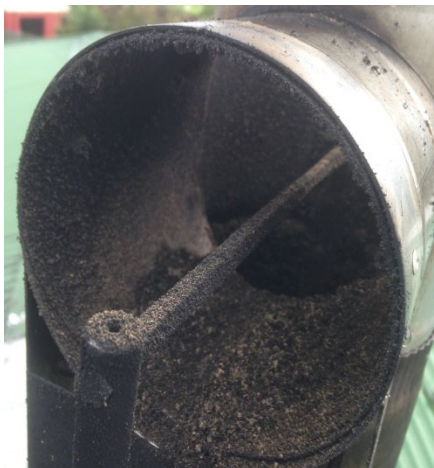
Black coal soot 1-4mm thick on upper flue wall, wall, 0.1mm on electrode, 27 June
