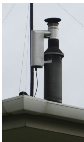
OekoTube circuit box on chimney
