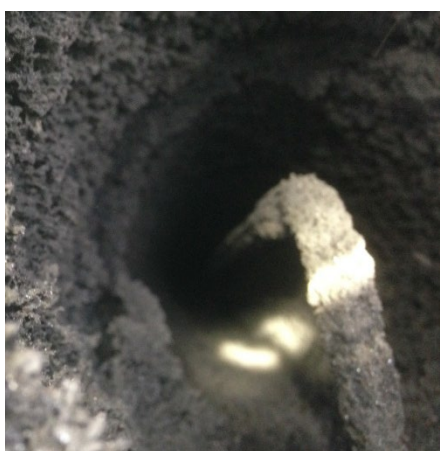
Wood-coal soot, less than ¼ the distance between the lower flue wall and the bottom of the electrode, grey/black colour, 27 June
